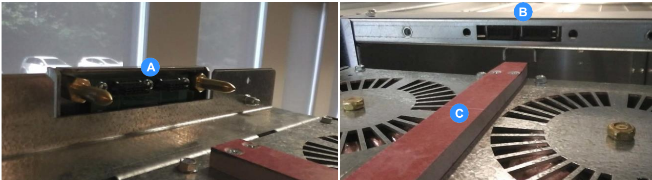
Figure 2.21 UPS module parallel bus connectors
